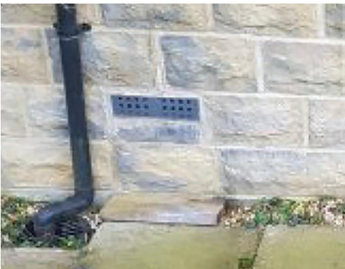
Waterproof render on the bricks and self-closing air bricks to reduce the entry of flood water
